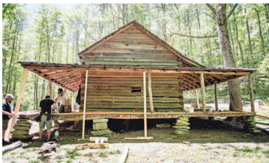
The Hands of Sean Perry Co. onsite during the 2017 project to shore up the floor joists and porch of Cook Cabin in Little Cataloochee, Great Smoky Mountains National Park.
