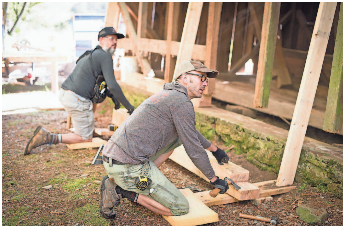
Crew member Rob Moody and company president Sean Perry work on the exterior of Palmer Barn during the 2018 restoration project of the iconic barn in Cataloochee, Great Smoky Mountains National Park.
